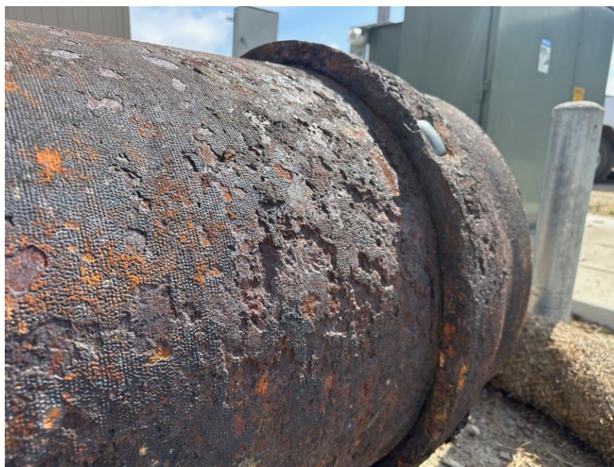
Figure 2-4. Corroded segment of ductile iron pipe removed per Xylem's dig sheet recommendations - Photograph 2 of 2
