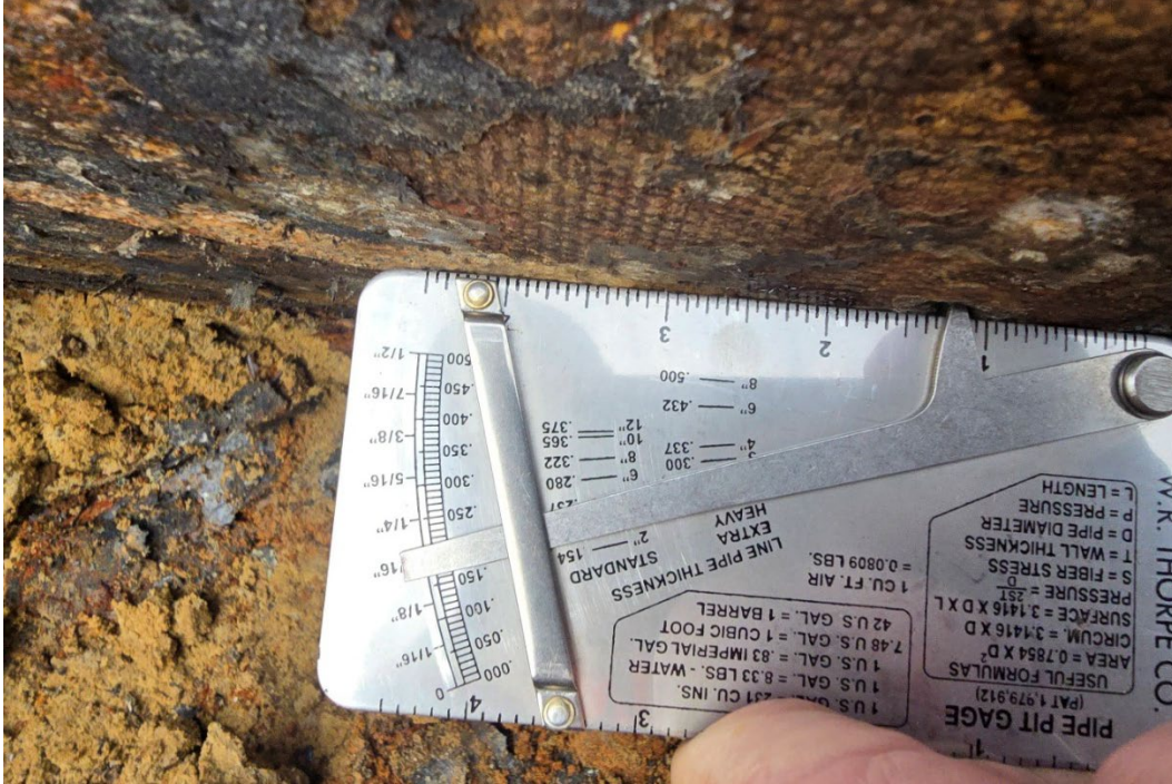
Figure 6. 0.150 inch pit found at STA 71+00
