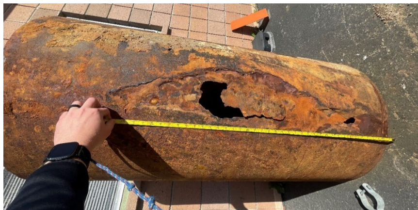
Figure 7: Failure section of the pipe
