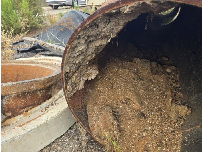
Figure 5: Solids accumulation in pipe invert (now seen in 10 o'clock position)
