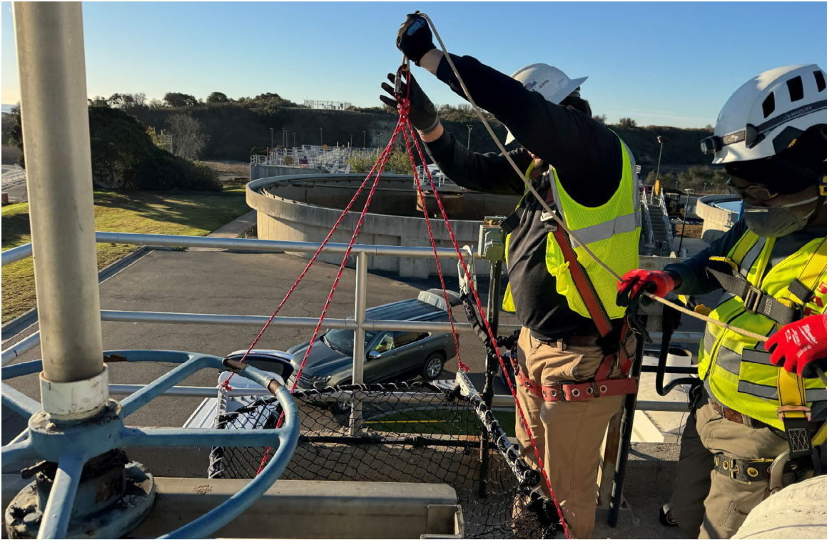
Figure 2.2: SmartBall Extraction Net Being Placed into Position
