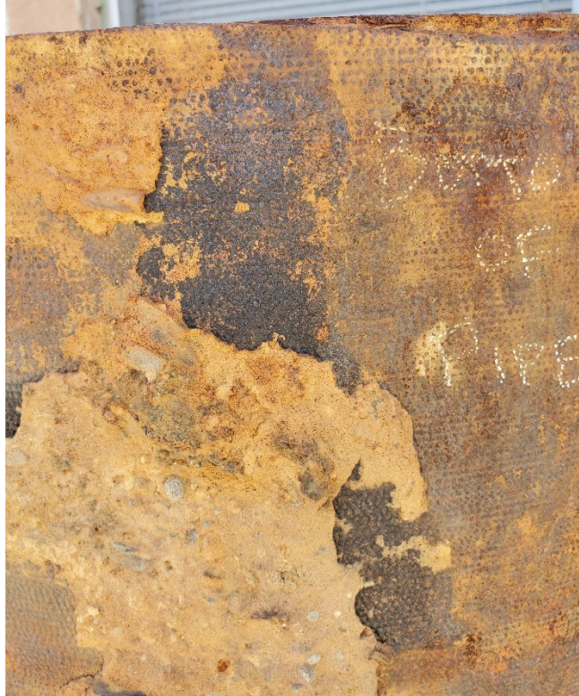
Figure 6: Encrusted scale with embedded aggregate
