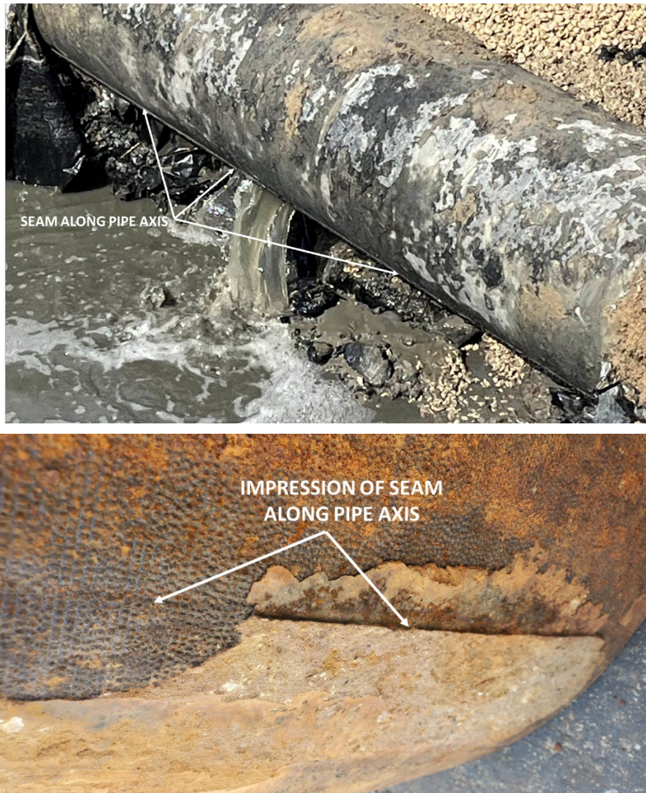
Figure 5: Photos suggesting a seam along the pipe axis, near the failure
