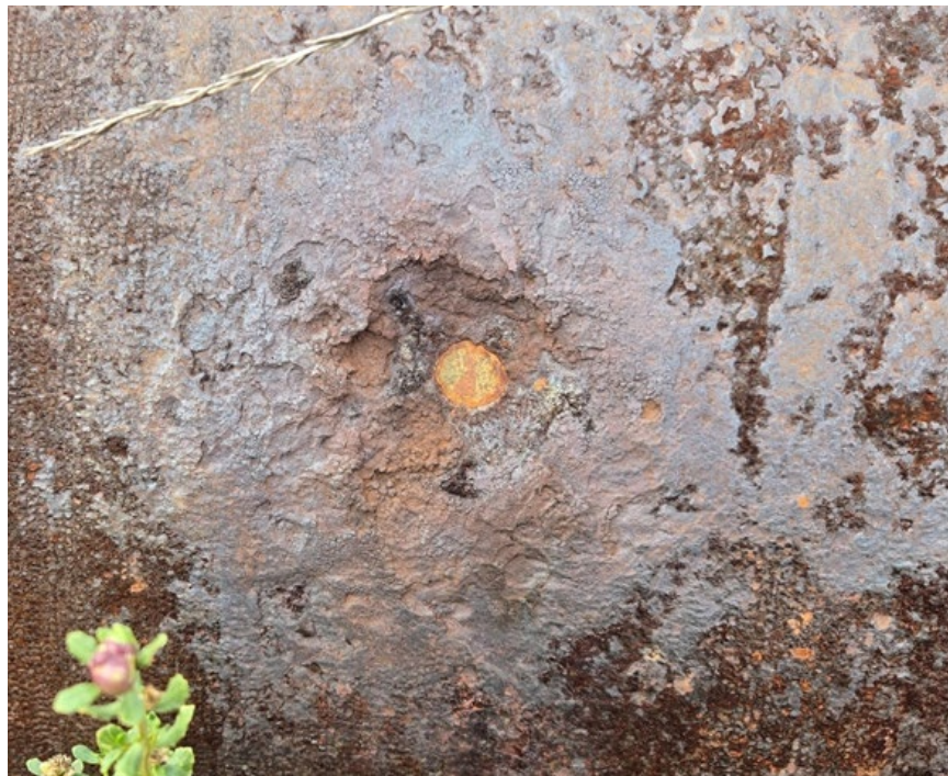
Figure 2: Corrosion through-hole at Pure's "Anomaly Area"
