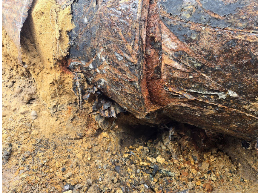
Figure 6: Corrosion near pipe bell at STA 69+50
