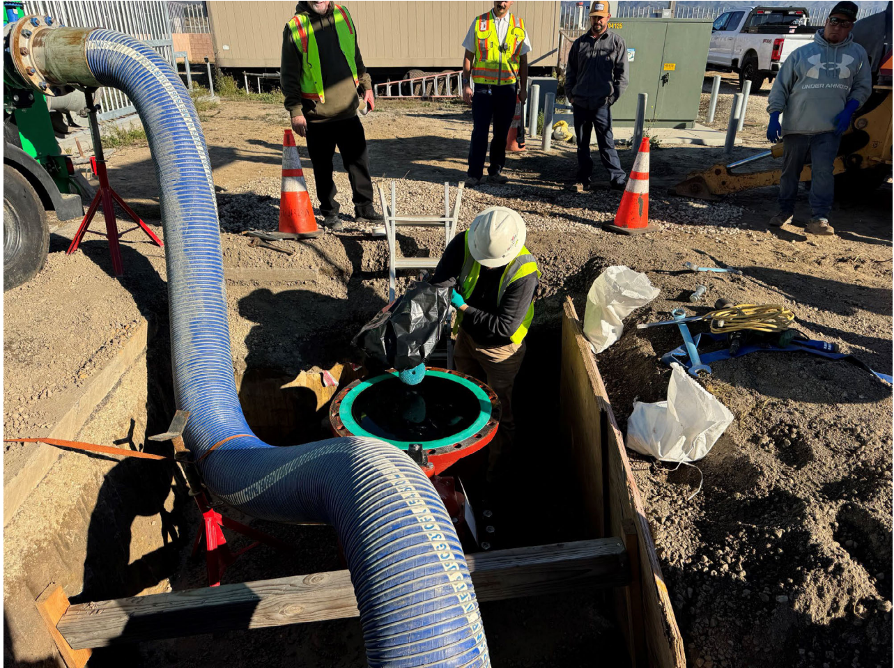
Figure 2.1: SmartBall Tool Being Placed into 24-inch Blind Flange at GWSD Yard
