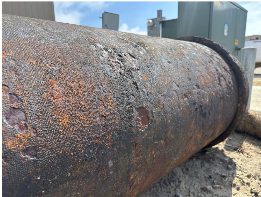
Figure 2-3. Corroded segment of ductile iron pipe removed per Xylem's dig sheet recommendations – Photograph 1 of 2.
