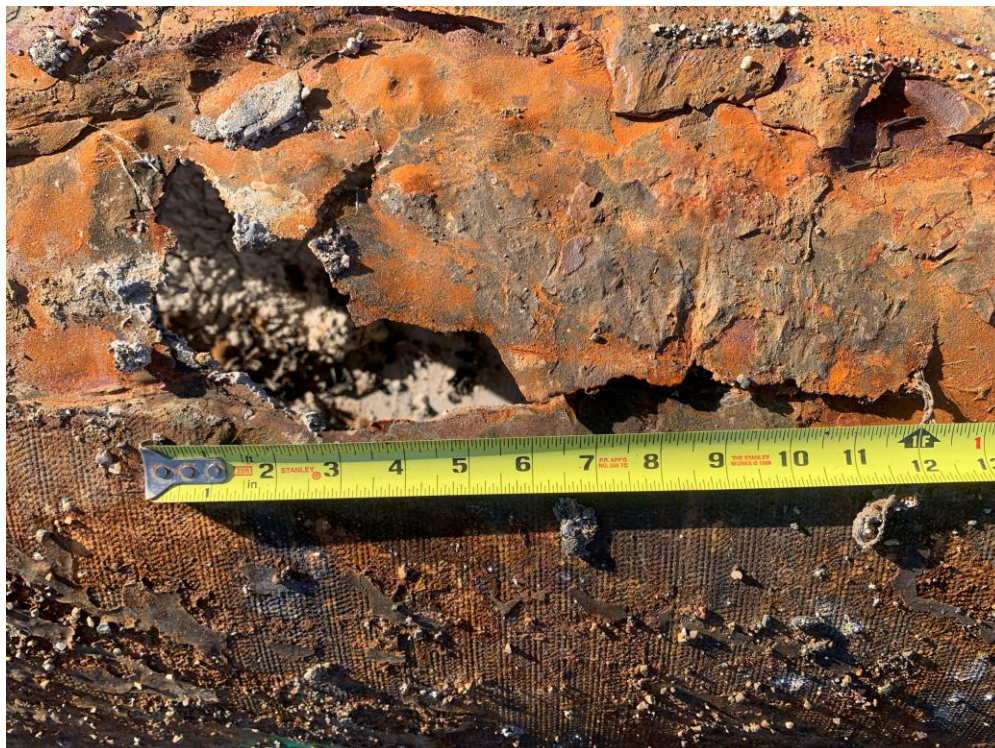
Figure 1-2. Ductile iron pipe section removed from the February 2024 spill site. Entire sections of pipe wall had deteriorated, revealing the inside of the pipe behind.
