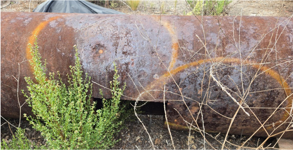
Figure 3: Corroded pipe in vicinity of Pure's "Anomaly Area"
