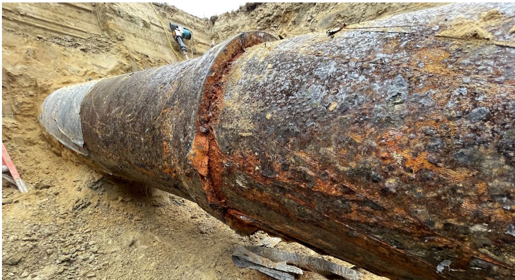
Figure 7: Corroded bell and spigot at excavation east of Moffet Place
