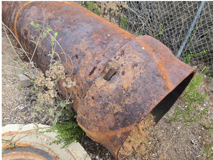
Figure 4: Through-hole at pipe joint
