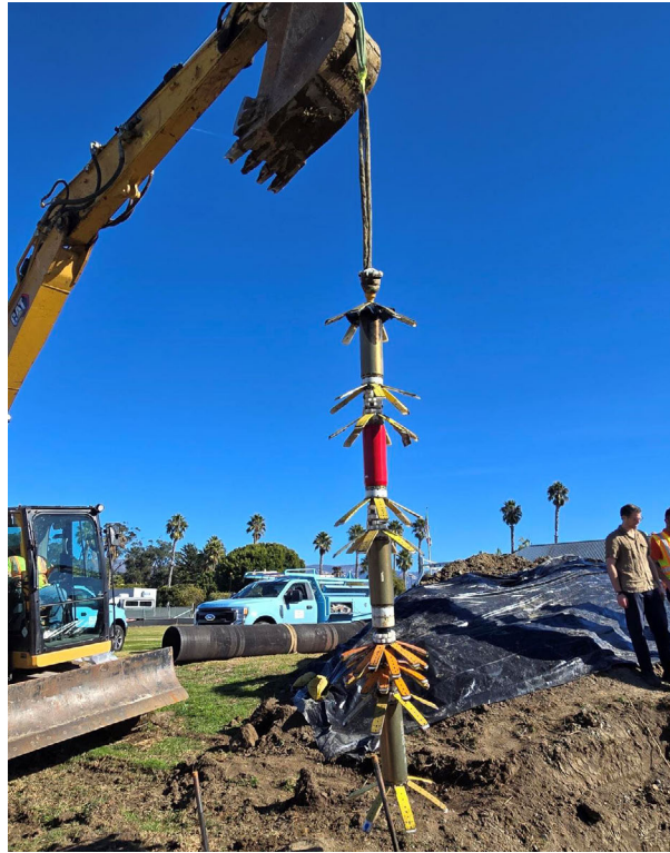
Figure 1.2: PipeDiver Inspection Platform Being Pulled from Pipeline
