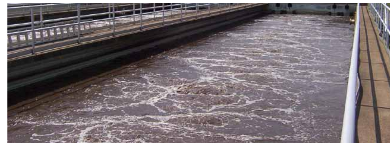
Secondary Treatment Tank
