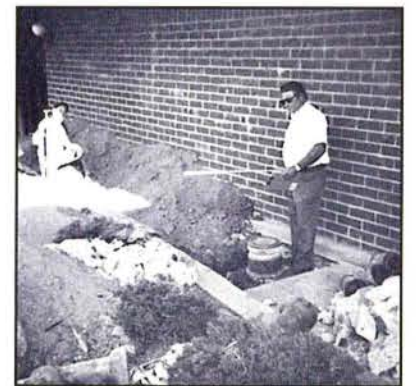
Larry Bales inspects a sewer replacement as part of his job as District Inspector.
