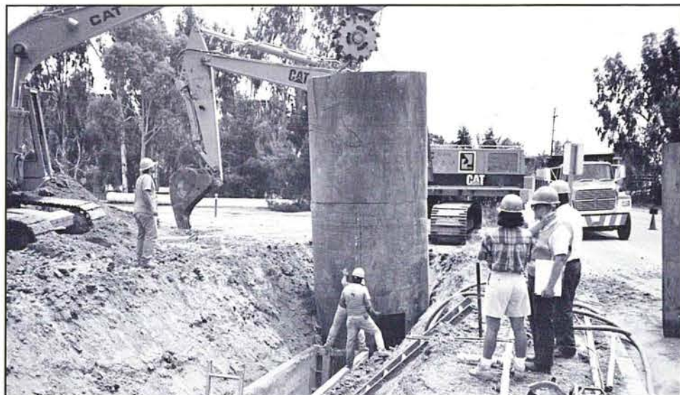
Steel pipe is being lowered into a drilled shaft for shoring during manhole construction in Los Carneros Road.
