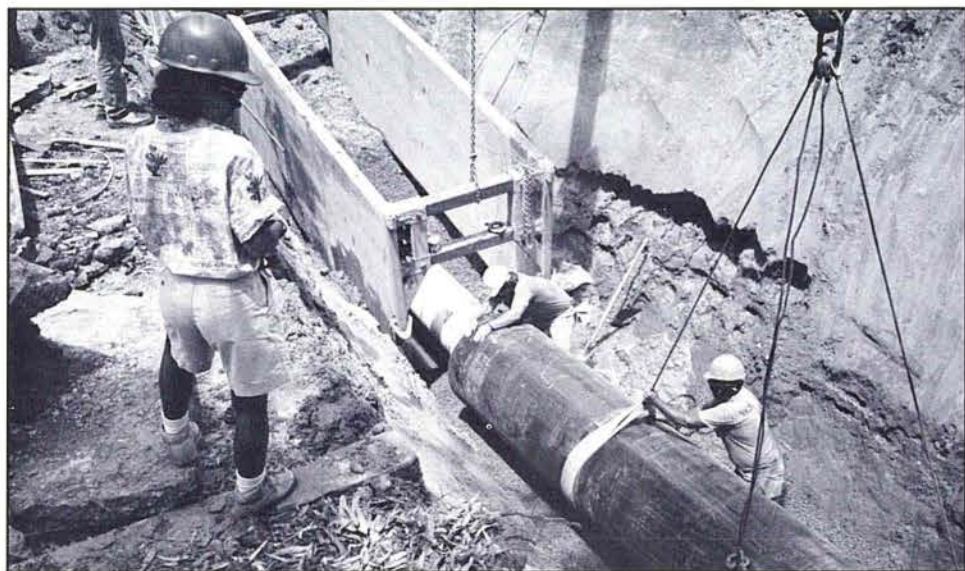
20" PVC pipe and a 36" diameter casing is being set in a trench in Los Carneros road.
